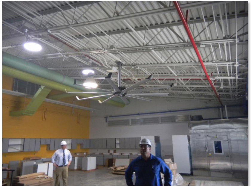
Interior space with fan, solar tubes, solar thermal heating
