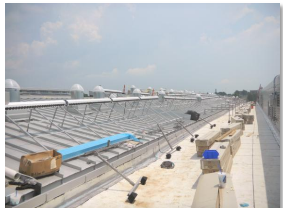
Rooftop solar thermal installation and exterior view of solar tube domes
