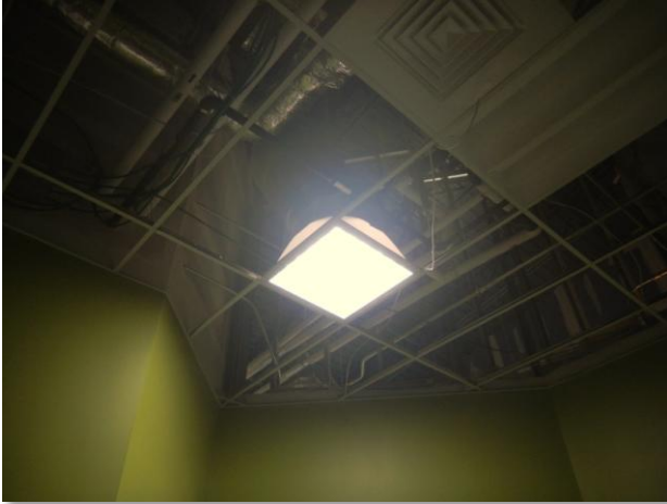
Interior view of solar tube used for daylighting
