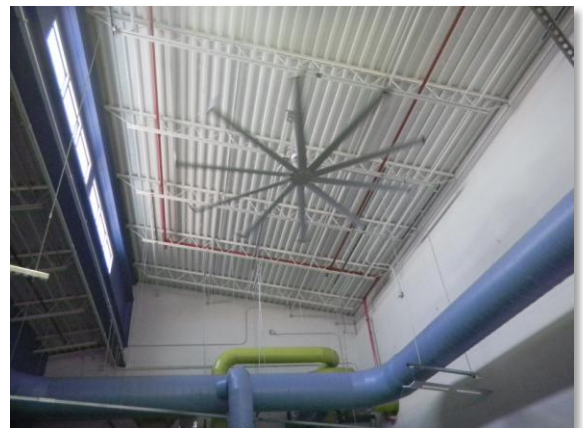
Big Ass Fan for air circulation, clerestory windows for daylighting, and HVAC ductwork
