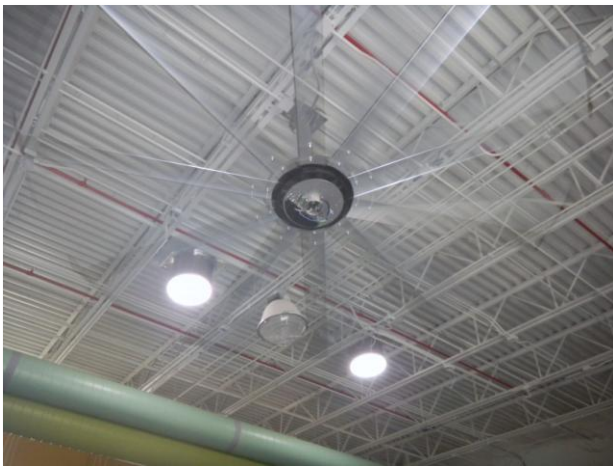
Big Ass Fan in action – energy efficient air circulation
