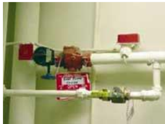
Sprinkler zone control station and zone indicator sign.
